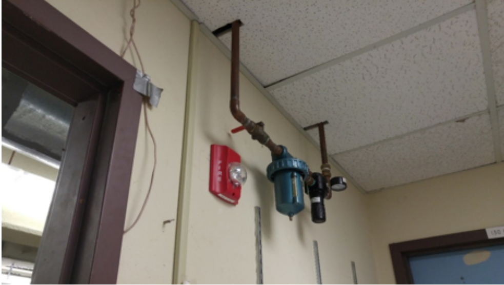
Off: the red handle is perpendicular to the pipes
