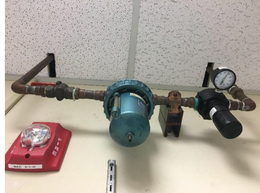
Figure 2: Main Air in the “On” position. Notice that the air pressure is around 90 psi.
