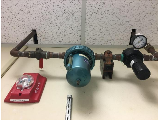
Figure 1: Main Air in the “Off” position. Notice that the air pressure is 0 psi.
