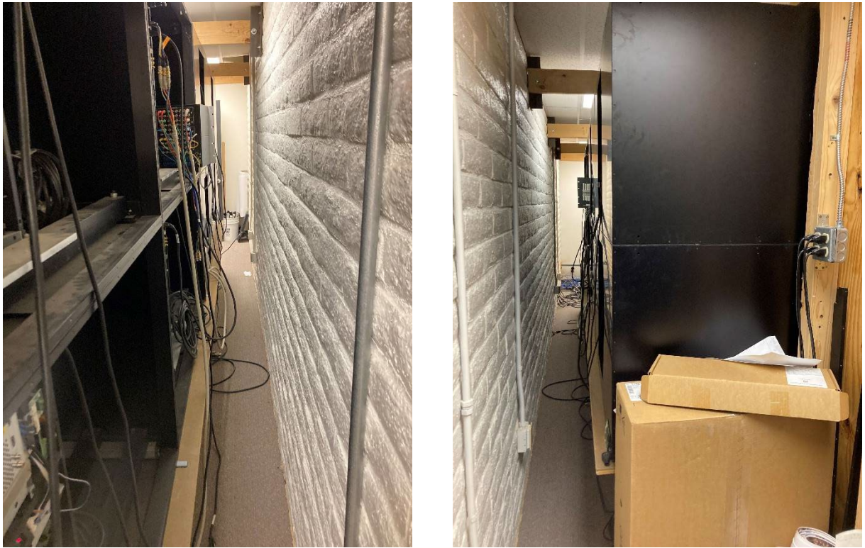
Figure 7: Network and electrical wiring/cabling behind the temporary wall supporting the current video screens
